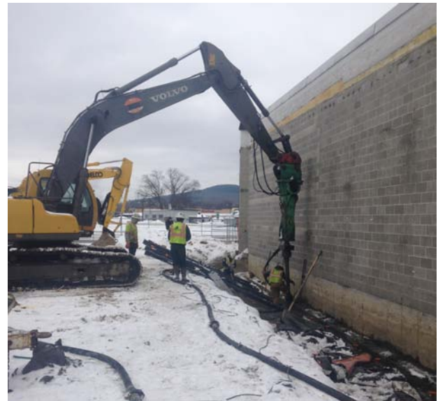
Figure 4. Picture of Installation Adjacent to Building
