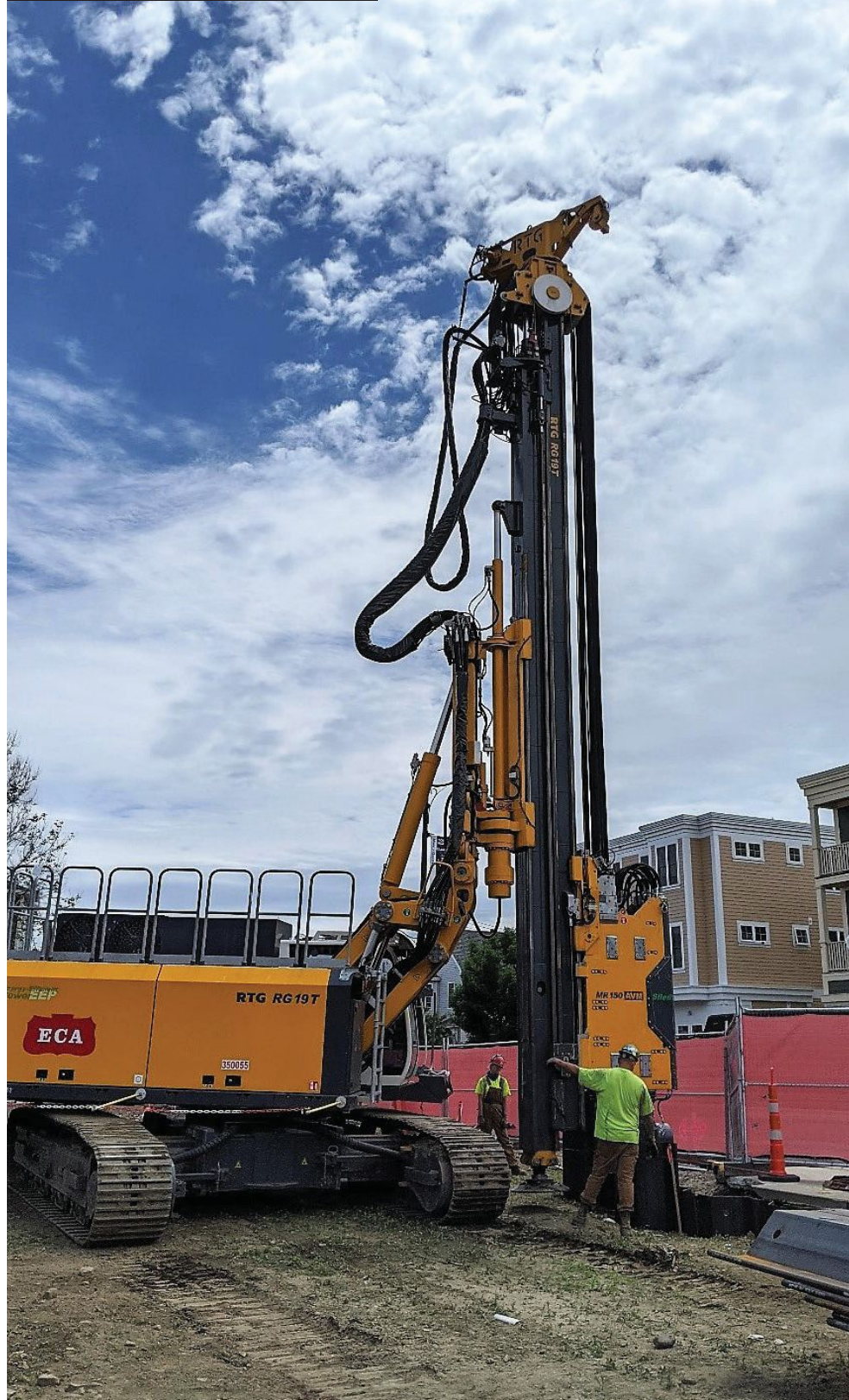
Keller North America used an RTG RG 19 T Piling Rig to install 40-foot sheet piles for SOE in Somerville, Mass. Photo credit: Equipment Corporation of America (ECA).
