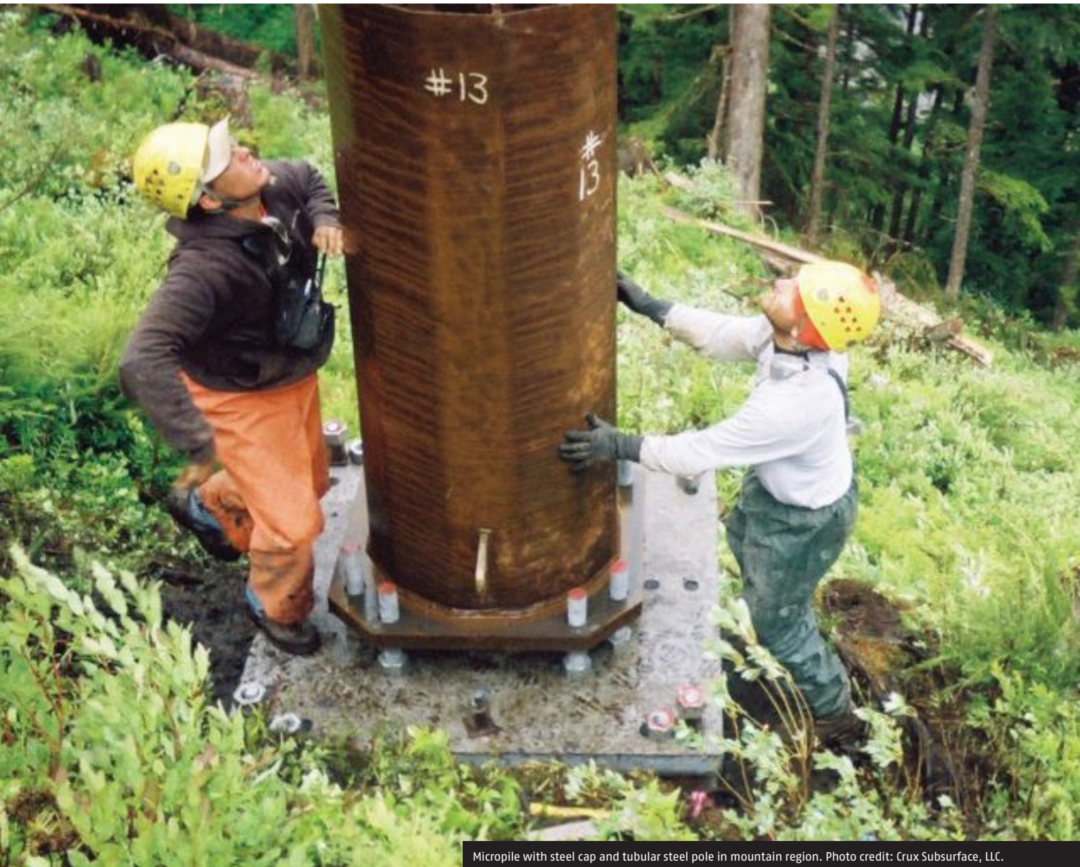
Micropile with steel cap and tubular steel pole in mountain region. Photo credit: Crux Subsurface, LLC.
